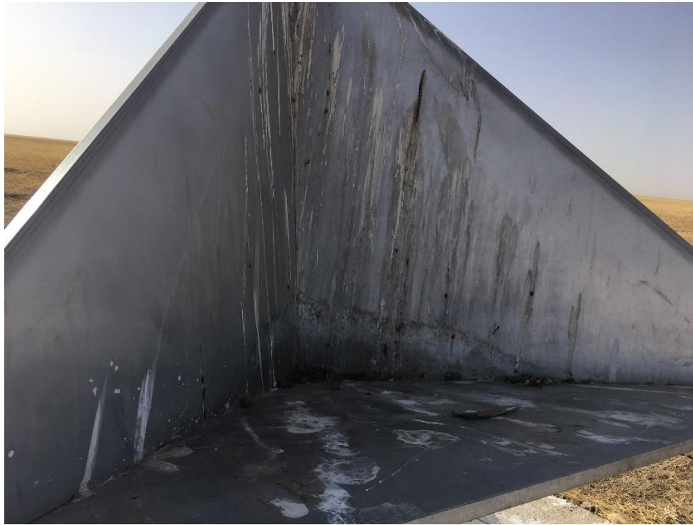
Aging of the surface condition
